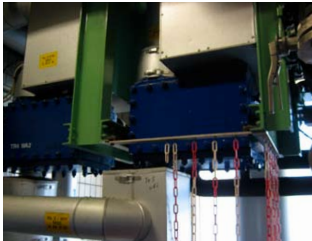
Suspended from the ceiling, the compact Alfa Laval Compabloc units save space at the Lanxess plant
